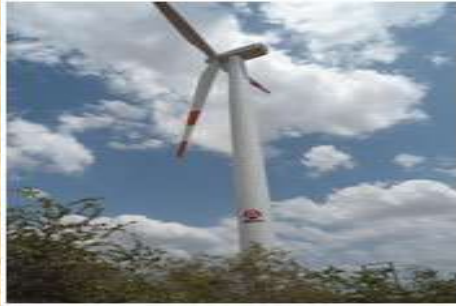
WIND POWER PLANT
