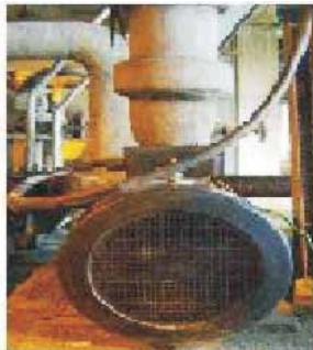
Replacement of old inefficient Secondary air conditioner pump1 with energy efficient pump1
