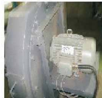
Provided interlock to stop the Dust blower when machine is not running
