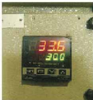
Temperature control of pm2 VAM Cooling basis fan resulting into energy saving in fan and additional pump(22kw) both.
