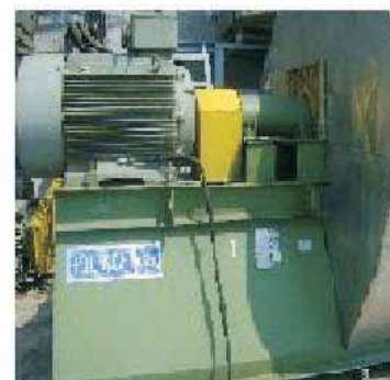
Stoppage of 1 No of Supply blower in coater 1 and coater 2 in PM2
