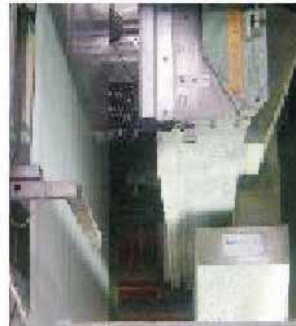
Stoppage of Pre-coat(1 &2) IR Drying system during all 180 GSM and above board paper in OMC
