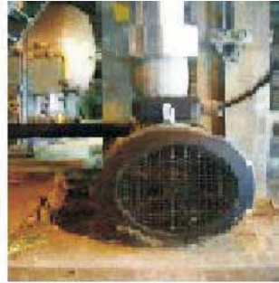
Replacement of old inefficient secondary air conditioner pump2 with energy efficient pump 2
