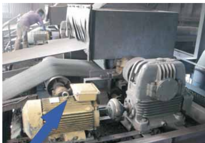
Downsizing of 22 KW motor to 15 KW
