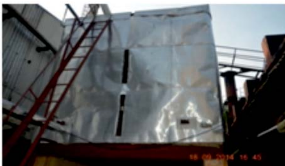
Condensate Heat Recovery
