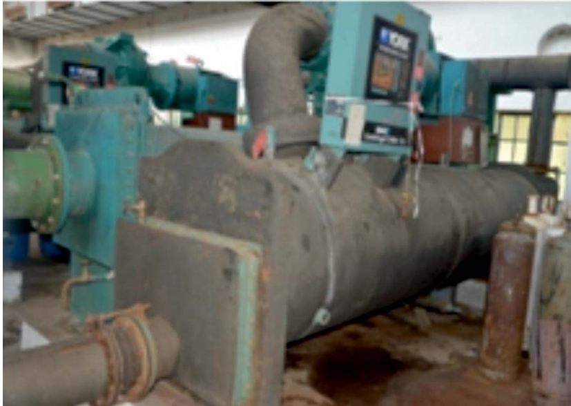
Shut down of 660 TR Chilling Unit
