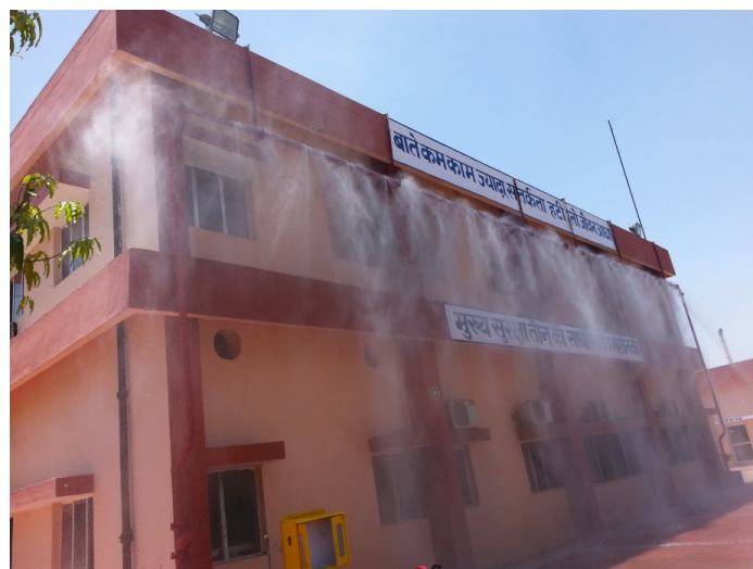
WATER CURTAIN FORMATION FOR FIRE PROTECTION
