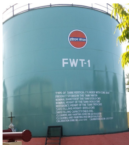
FIRE WATER TANKS
