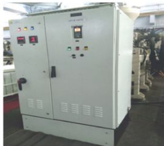
After VFD Installation
