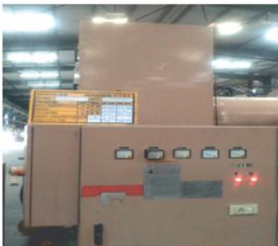
Before VFD Installation
