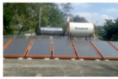
1000 LPD Solar Water Heater at Running Room, Raichur
