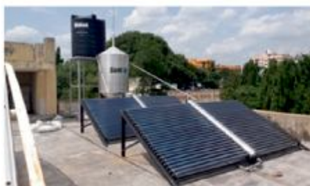
1000 LPD Solar Water Heater at IRISSET/SC
