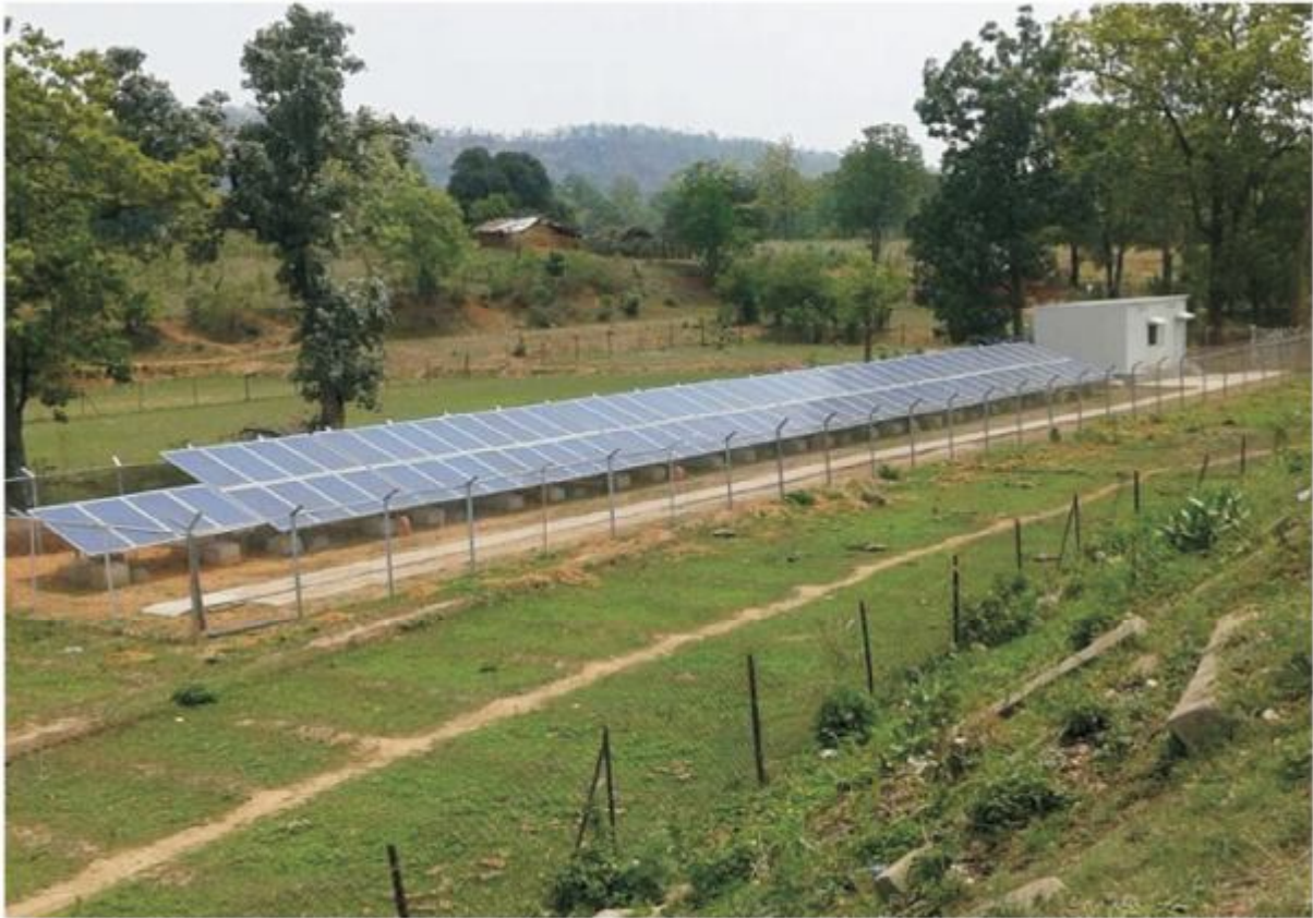
25KWp Solar Power Plant at Bhanwartonk
