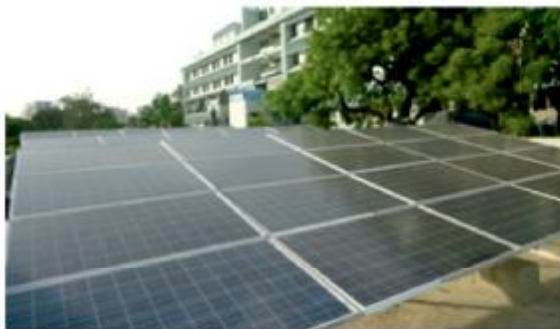
10 kWp ON grid Solar Plant at Sanchalan Bhavan Annexe
