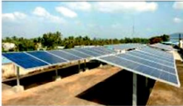
15 kWp ON grid Solar Plant at Anakapalli Station
