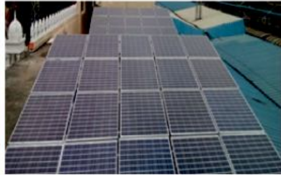
15 kWp ON grid Solar Plant at Bellampalli Station
