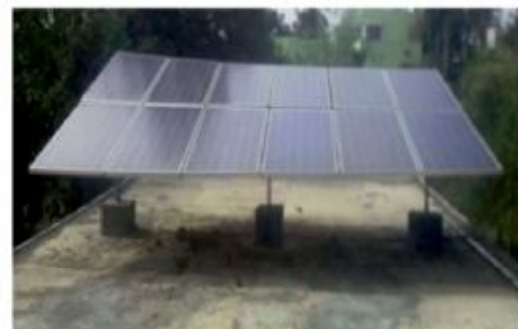
3 kWp OFF grid Solar Plant at Bidar Running Room
